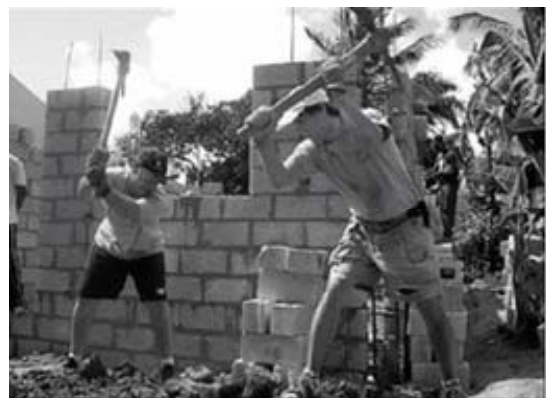
Craig Hlavac and Chris Mayes, both of Wallingford, work on the school Friday.
