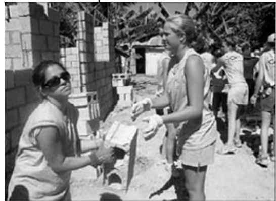
Karen Grunwald, 17, right, of Wallingford, hands a concrete block to Brittani Piekarski, 16, of East Haven. They are building a computer school in rural Dominican Republic.
