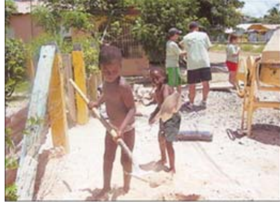
Two young Haitian boys help move sand Friday for the cement that's being used to build a computer school at Batey La Higuerra in La Romana, Dominican Republic.
